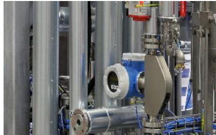
System components (pumps, pipes, etc.)
